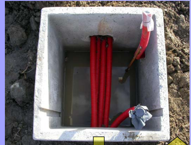
Underground cable tubes
