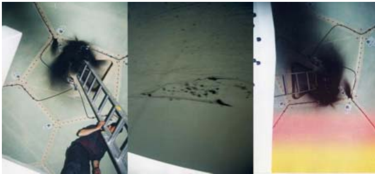
Some parts of radome damaged by lightning strikes
