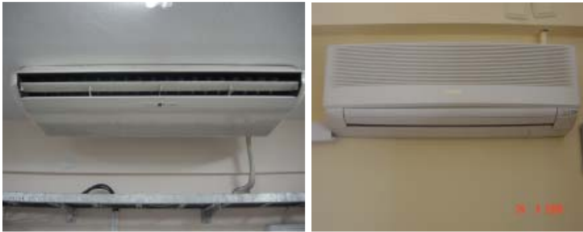
Figure 15: Heating and Air Conditioning Systems.
