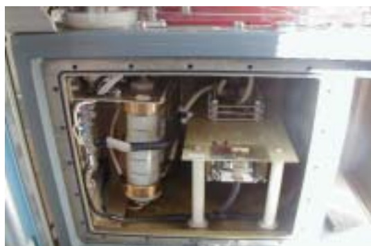
Figure 33: Inside of an Air Isolated Tank.
