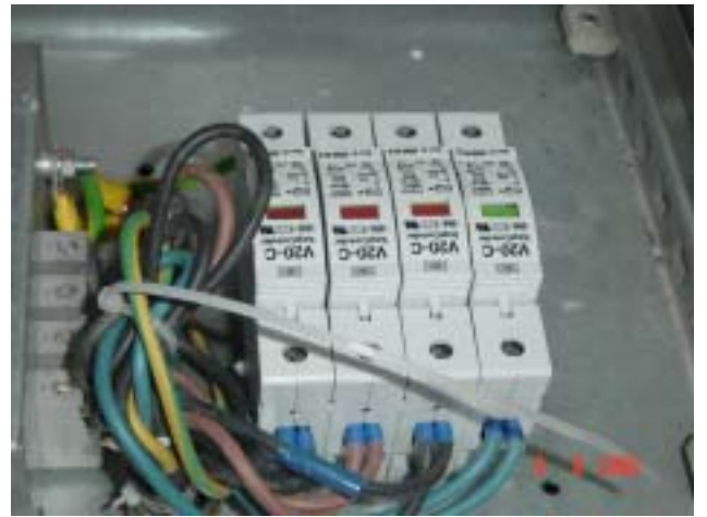
Figure 7: Some Lightning and High Voltage Protection Pictures.
