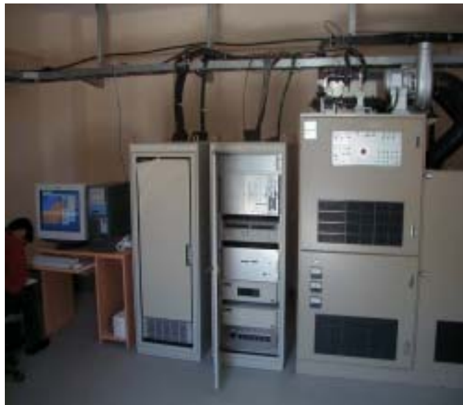
Figure 59: Hardware of Zonguldak Radar/Turkey.
