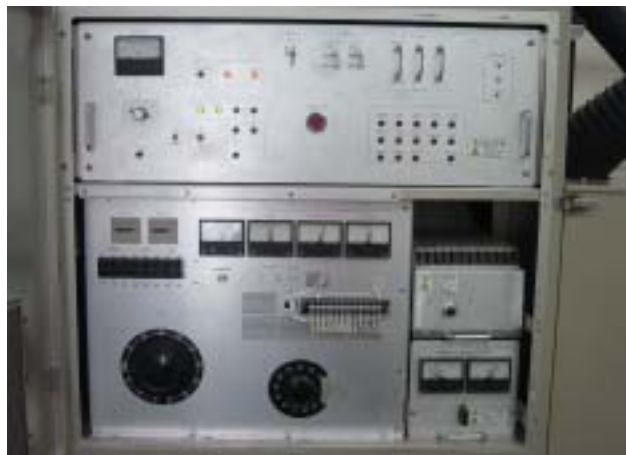
Figure 26: Front Panel of a TX Cabinet.
