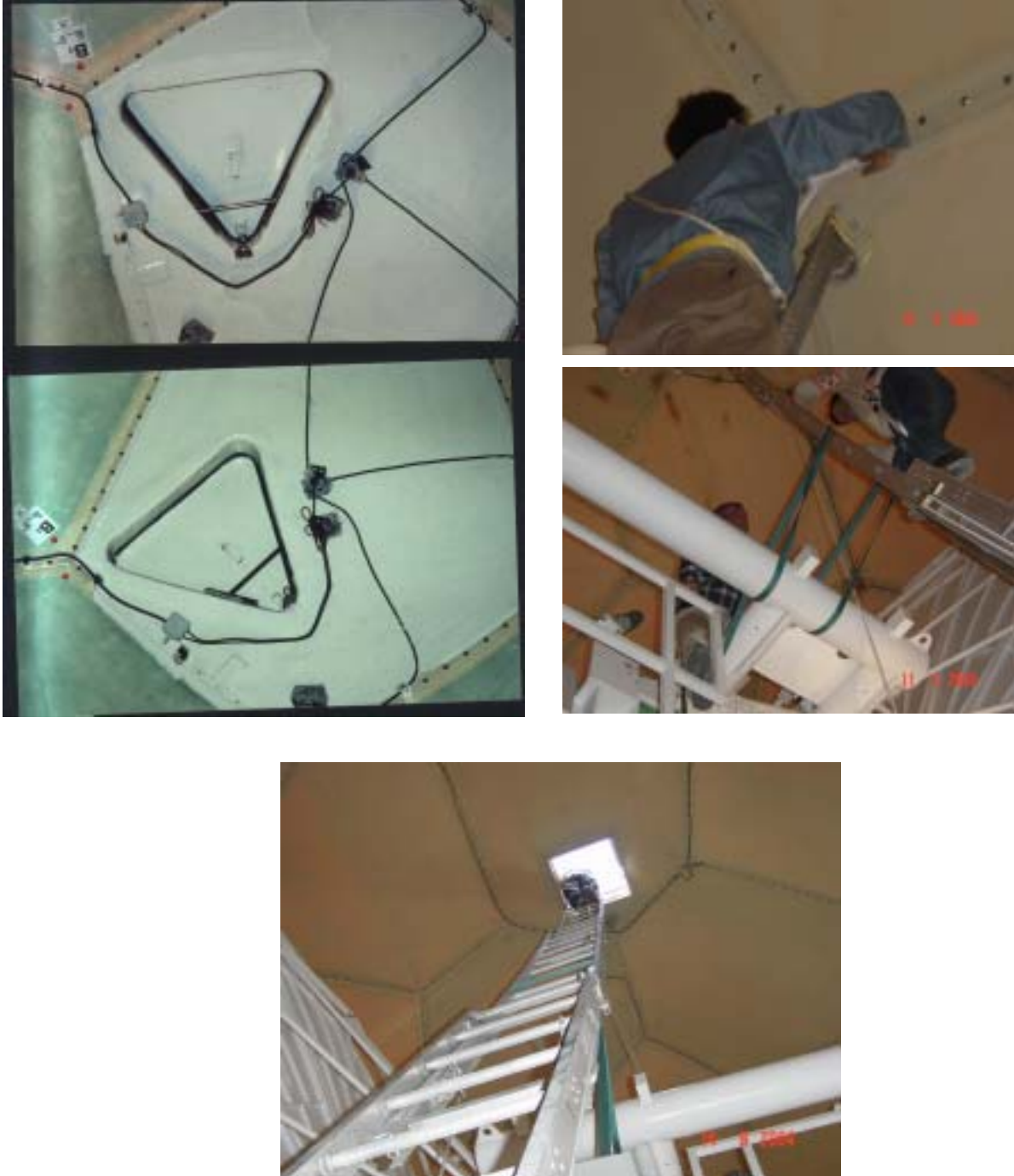
Figure 42: Obstruction Light and Lightning Rod Connections on Radome, Applying Silicon to the Leakage and Changing Obstruction Light.
