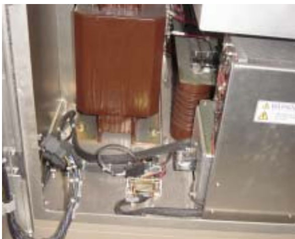
Figure 28: High Voltage Section of a TX.
