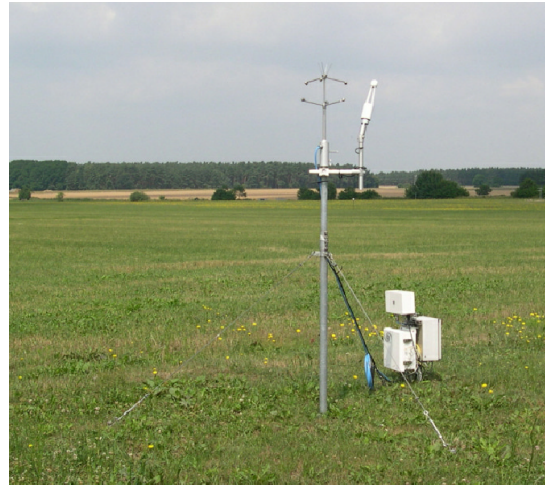
Figure 2: field installation (LI-7500, USA1)
