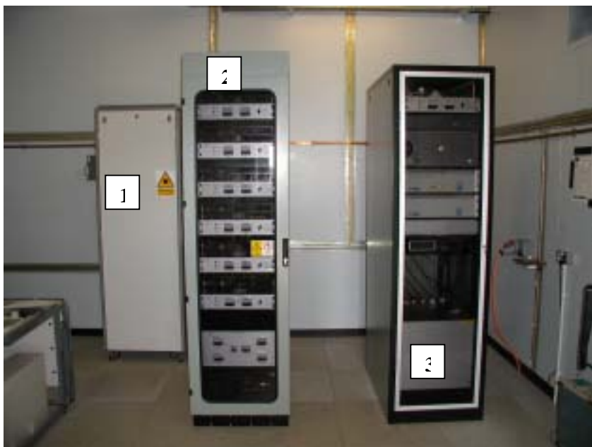
Figure 7 – Internal Electronics. (1) Communications cabinet. (2) Transmitters and power supply. (3) Beam Steering unit and digital processing.
