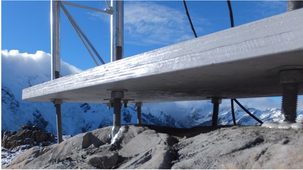
Figure 7: One metre threaded rod drilled and epoxied into bedrock with levelling plate.
