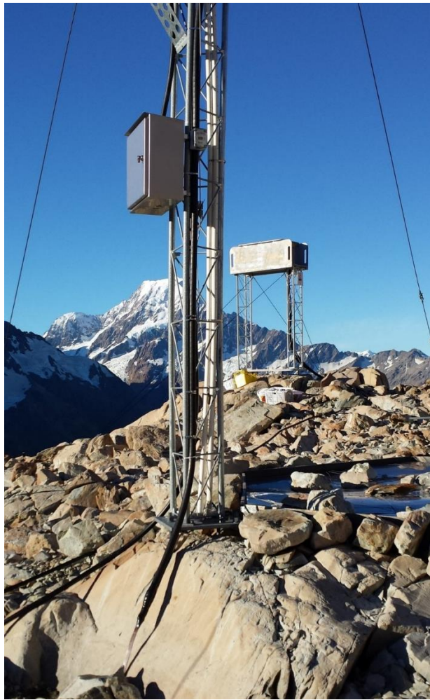
Figure 12: Earthing system, snow pillow, fuel cell housing and Aoraki/Mt Cook
