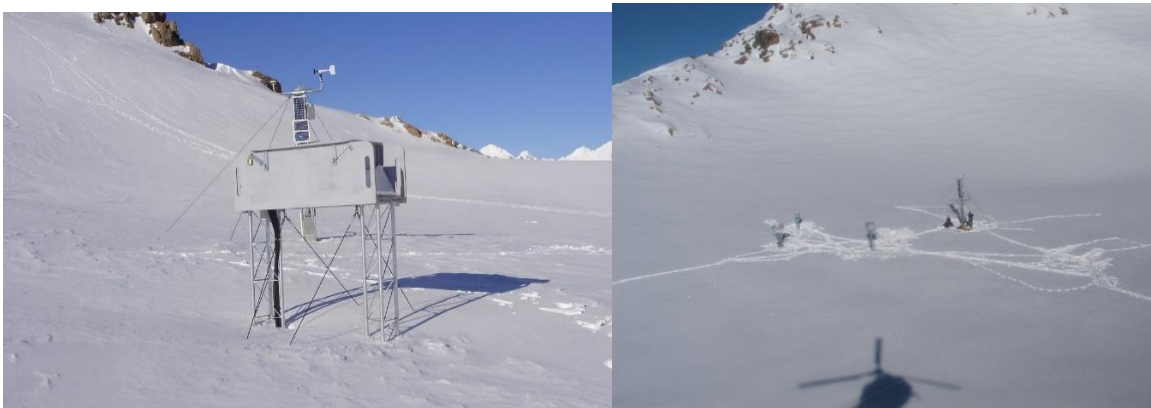
Figure 8: Enclosure for EFOY fuel cells and generator. EWS mast is visible in the background also. Overall layout of Mueller Hut site with 1m snow pack. Shielded gauge is to left.
