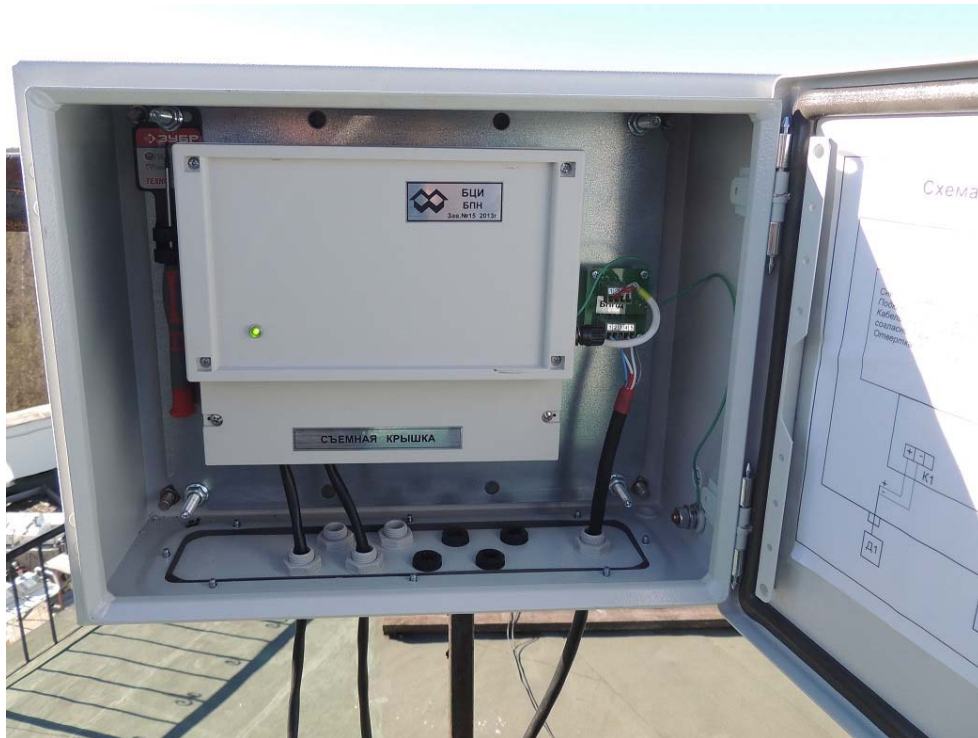
Fig.1 Central measuring unit (logger) in a weatherproof box
