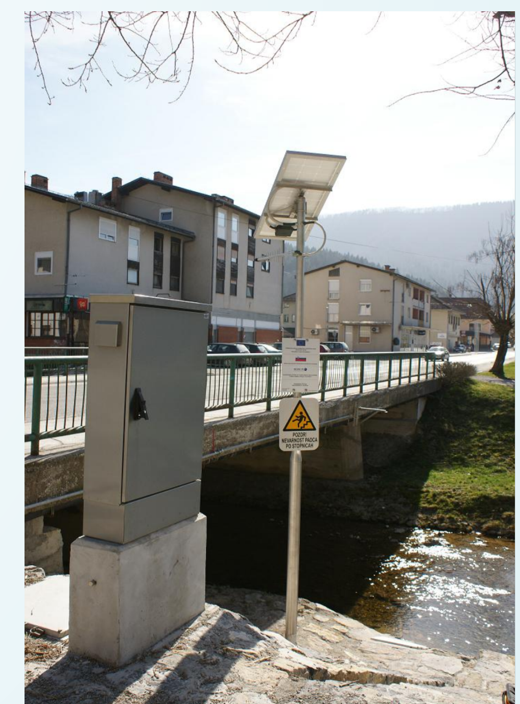
Figure 5: Photo of low power hydrological X-DEG based station at location river Bistrica Sodražica Slovenia
