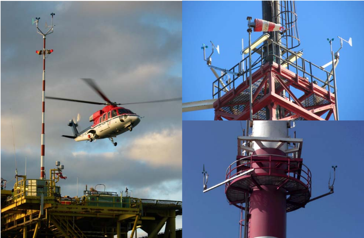
Figure 17: The wind measurements near the helideck of platform F3 (top left) and on the vent stack of K14 (top right) and AWG (bottom right).
