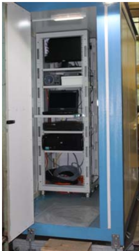
Figure 4 Inside view of the operator cabin.
