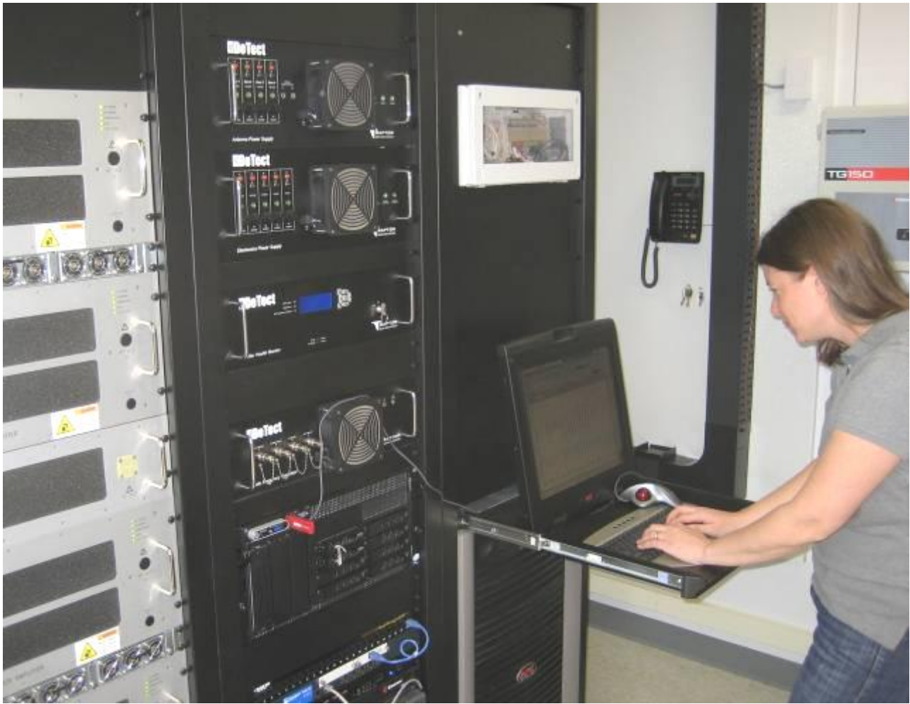
Figure 3: The RAPTOR transmitter is shown on the far left. The 2-kW modules can be seen along with the redundant DC power supplies. The antenna and electronics power supplies are shown in the top middle. Below these systems are the health monitor, the transceiver subsystem, and the wind profiler computer.
