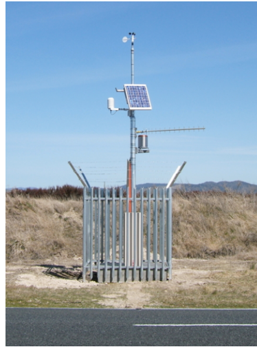
Road Weather Station
