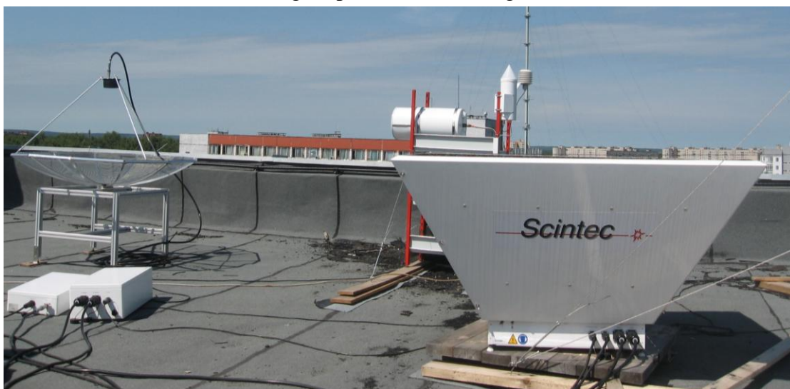
Figure 1 The photo of the equipment installed on the roof of the building 700 m apart from the tower.
