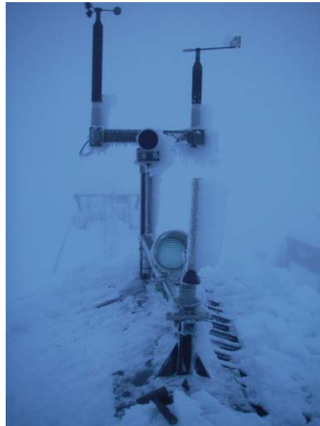
Figure A. 45 Pictures of the site installation in Åre on top of the roof of a ski lift house, with a camera mounted on the wind sensor support. The site is also prepared for remotely controlled de-icing of the sensor using
