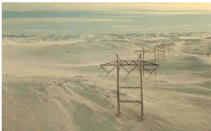
Figure A. 4 420 kV line crossing the mountain divide (1 100 m asl) between western and eastern Norway (Photo: S.M. Fikke)
