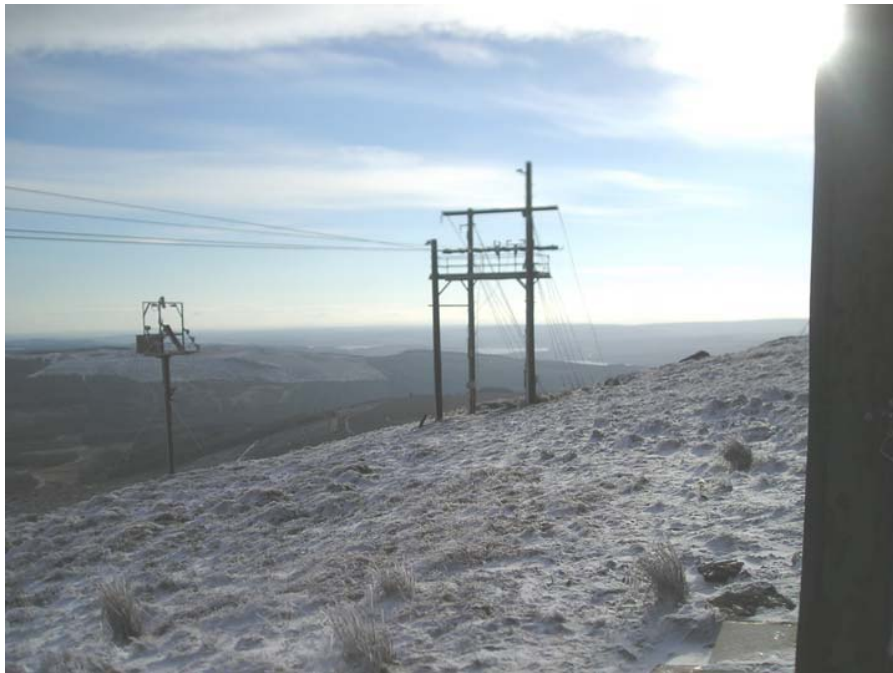
Figure A. 32 The Southern dead end platform and rotating rig at Deadwater Fell.
