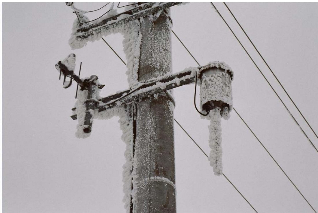
Figure A. 40 Device Meteo on a concrete pole of LV power line, location Predin (Photo: J.Sabata)
