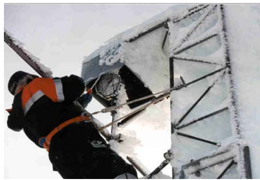
Figure A. 7 Details of dynamometer suspension in the rack
