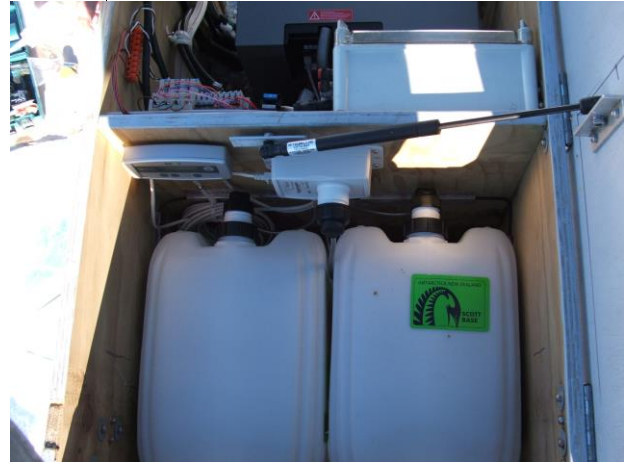
Photo 12: EFOY generator fuel cells (2x M28 Ethanol)
