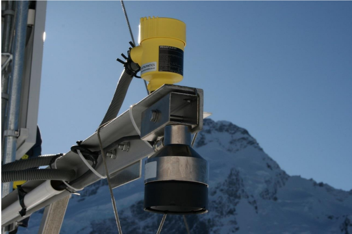
Photo 14: SR50A detail – Vega radar no longer used (December 2012)
