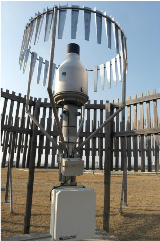
Photo of installation – Geonor gauge with Single-alter shield inside DFIR (South)
