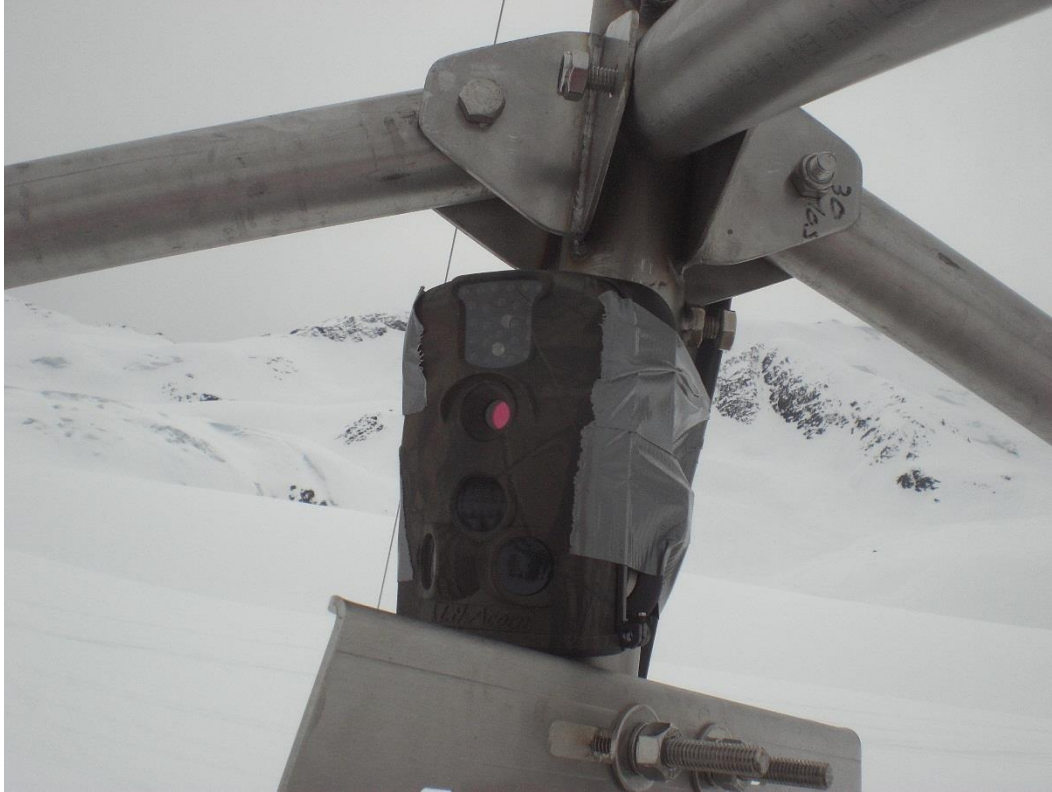
FIGURE 15: Detailed picture of the camera installed at the AWS Forni SPICE.
