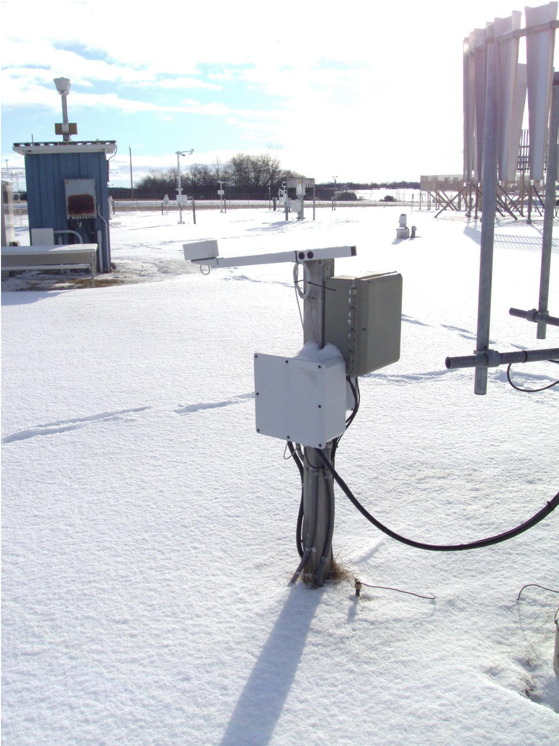
Photo of installation - precipitation detector
