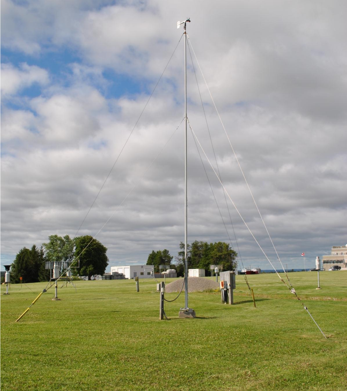
Photo of installation - R.M. Young Wind Monitor
