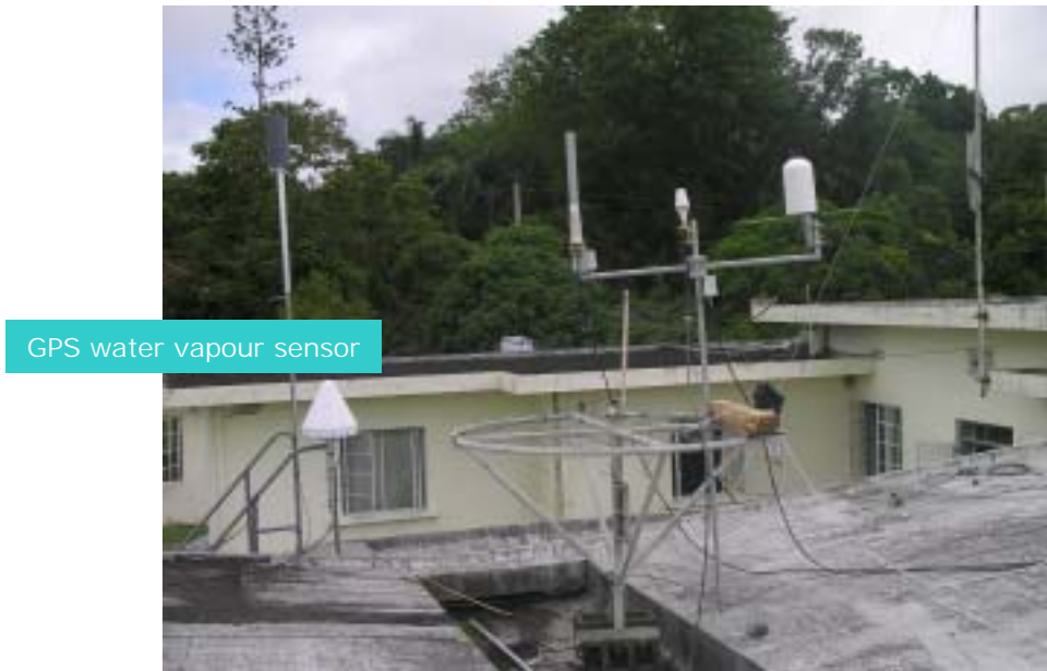
Fig. 12.1(b) GPS water vapour sensor installed on the handrails of the staircase to the roof, Vacoas.
