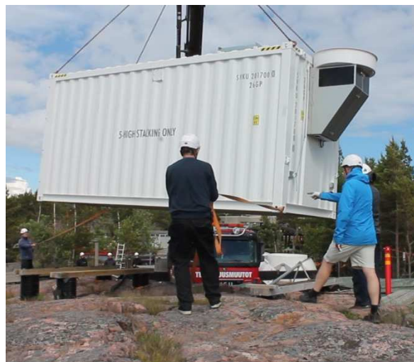
Figure 5. Installation of an automatic sounding station with the help of a truck equipped with a crane. Part of the balloon launch equipment has been installed at site, before lifting the container.
