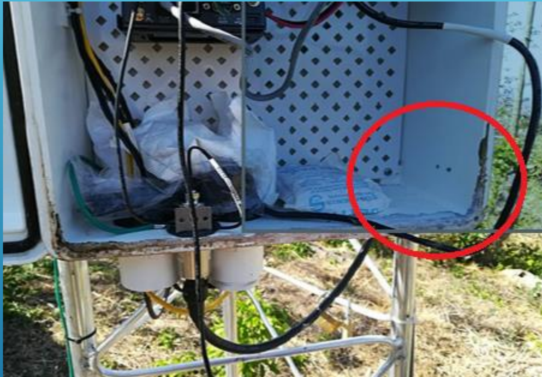
Acid spilled from the battery, damaging the fiber of the box.
