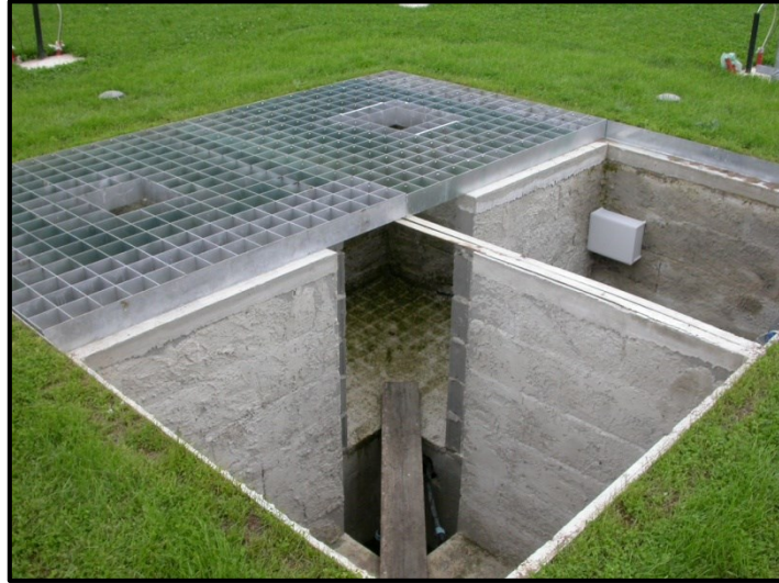
Fig. 5.6 The gratings, the pit internal walls and the pit recess for drainage (Vigna di Valle, Italy, 2007).
