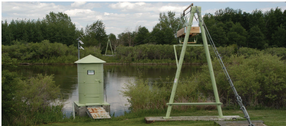
Figure I.2.2. Gauge with walk-in shelter, solar panels, satellite antenna, and cableway
