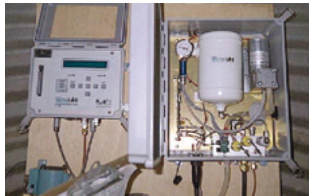
Figure I.4.26. Design Analysis Associates Model H-355 self-contained gas-purge system
