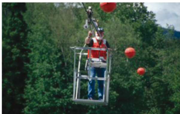
Figure I.5.48. Stand-up cable car in operation
