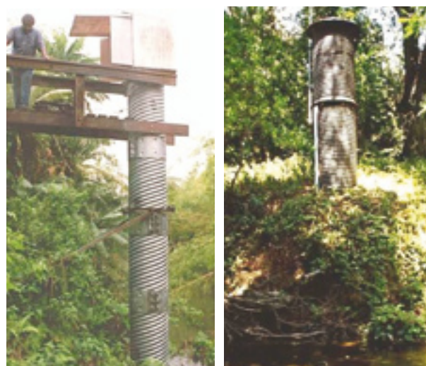
Figure I.4.2. Corrugated-galvanized-steel stilling well and shelter
