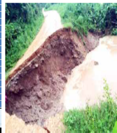
A section of the collapsed road linking Paktha to Huayxai districts in Bokeo province.
