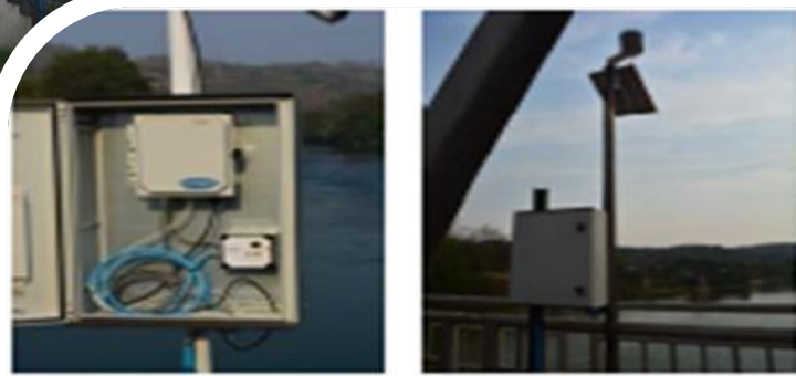
Install the telemetry system with Funded by Norway Gov.
