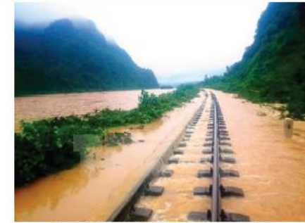
Many sections of the North-South railway have been affected by flood.
