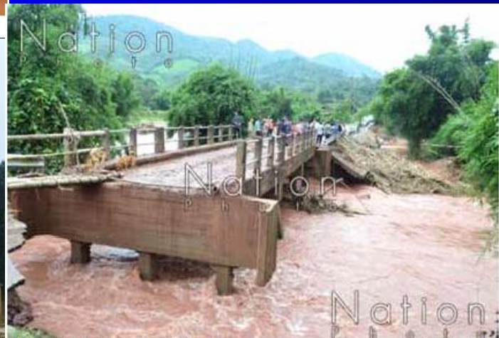
A bridge in Thailand hit by Tropical Storm Dianmu.
