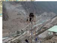
Punatshang Chhu 1 Power House Siren
