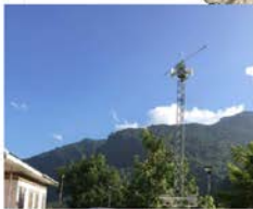
Siren at MHPA Power Plant
