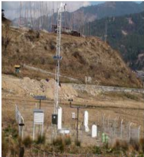
Photo 7: AWS installed at Chamkhar, Bumthang
