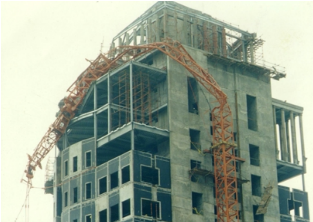
Figure 2 — Giant crane damaged by a tropical cyclone (Photo: Y. Boodhoo)
