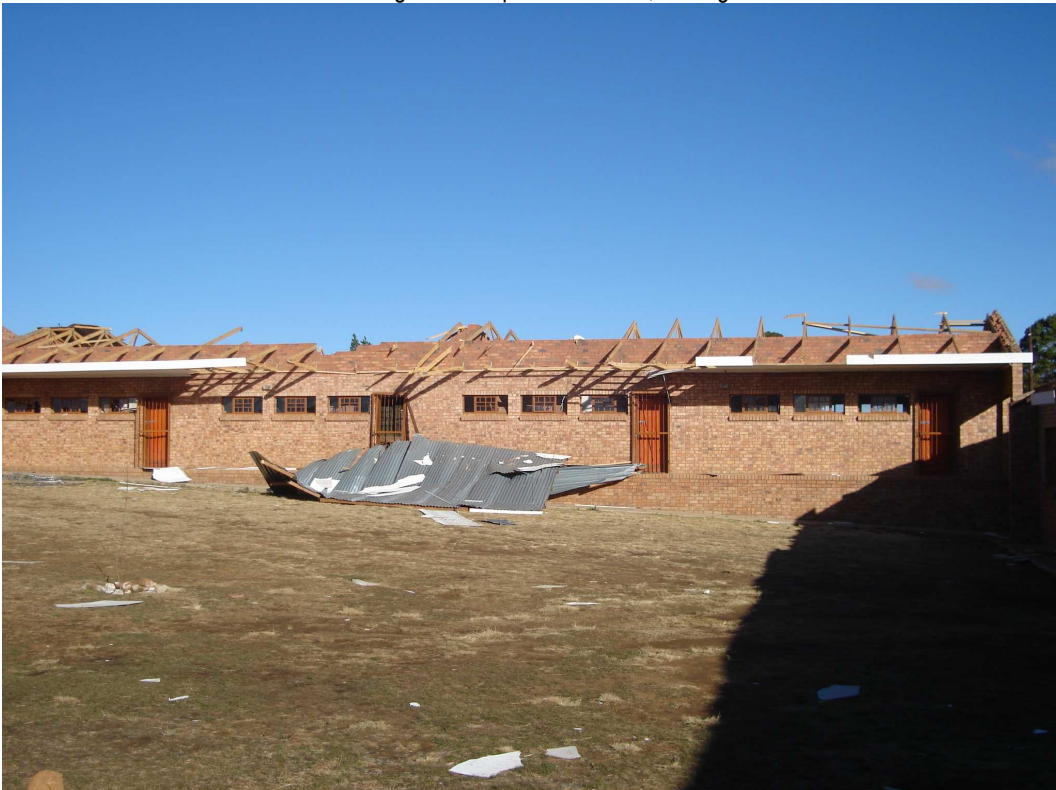
Tornado damage to a school at Dullstroom, 01 August 2006
