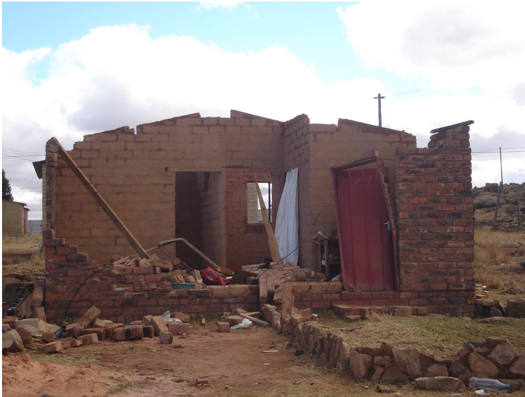
Severe damage to a township house outside of Dullstroom. Injuries occurred to the people in this house at the time of the tornado.
