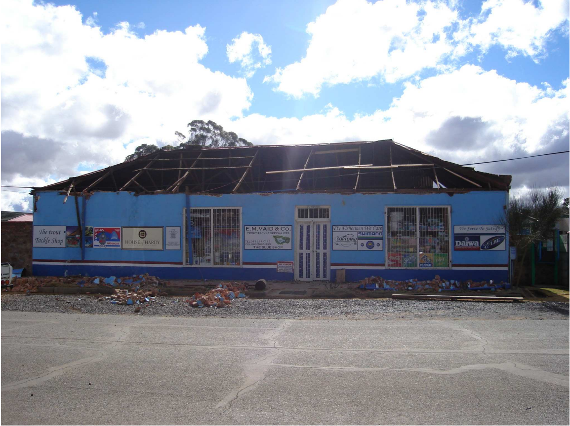
Tornado Damage to a shop in Dullstroom, 01 August 2006
