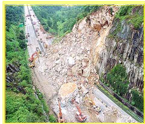
Fig. 6: Landslide along the North- South Expressway
