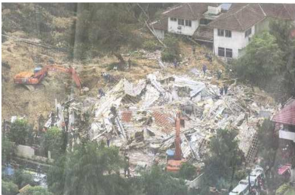
Fig.5 : An aerial view of the house in Taman Hillview that was destroyed in the landslide
