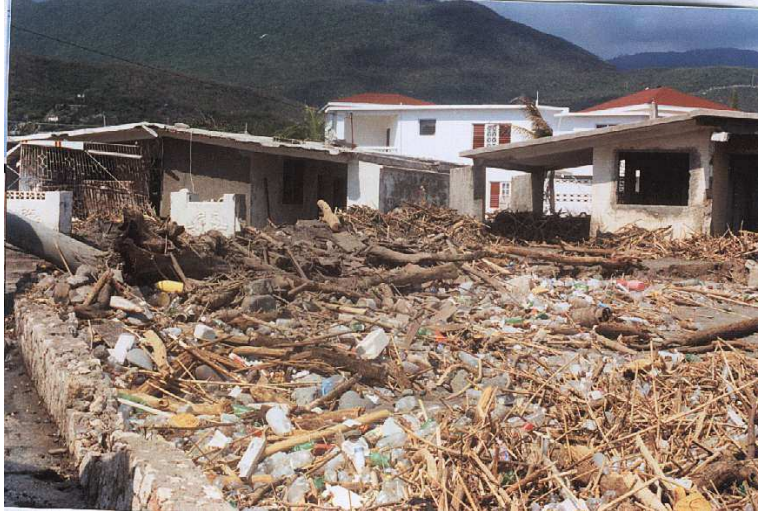
Plate 1: Severe damage to houses on the southern coast caused by storm surge associated with Hurricane Ivan in September 2004.
