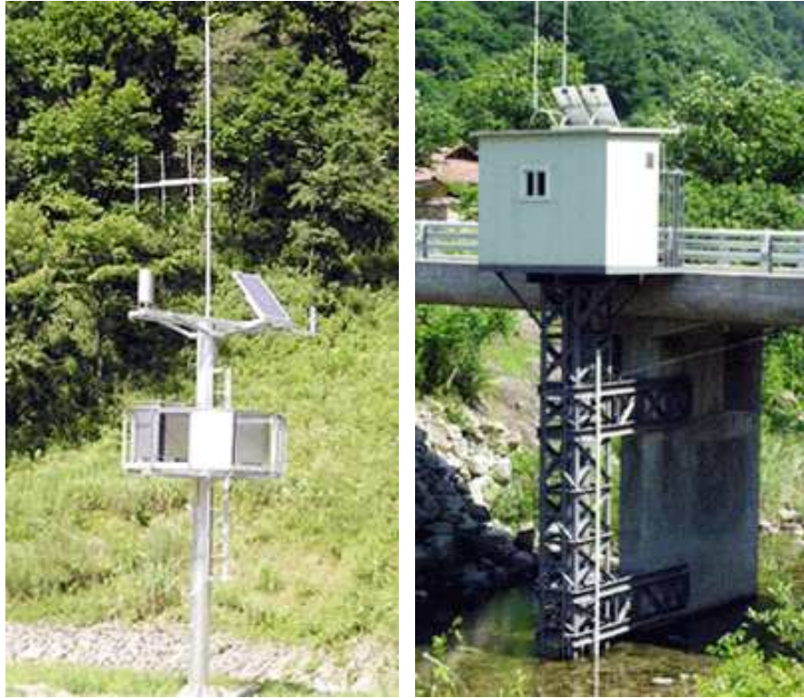
<Figure 1. Observation Station for the Rainfall Warning System>
