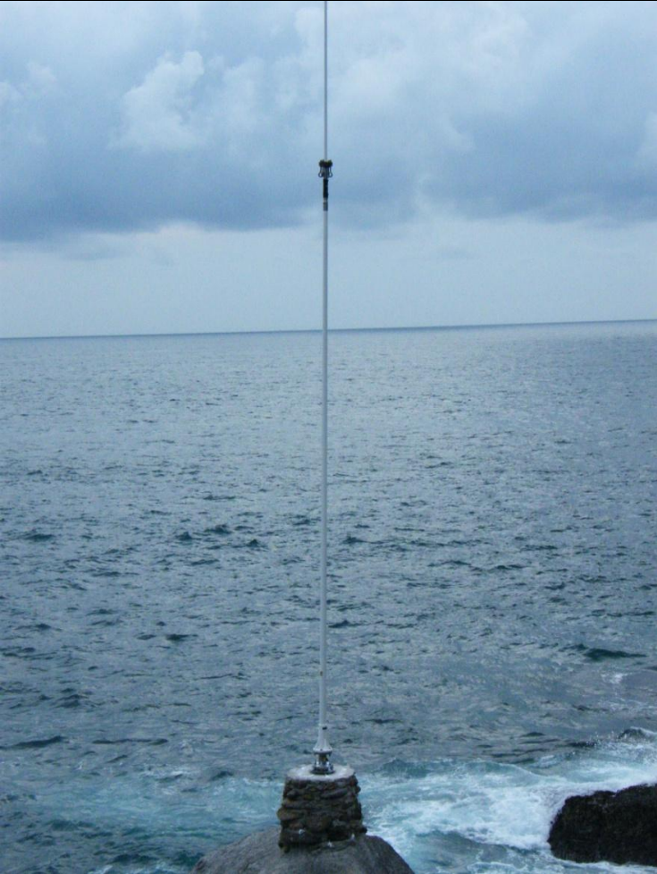
Transmitter at Phuket site
