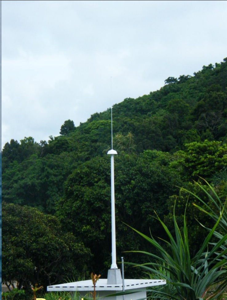
Receiver at Phuket site
