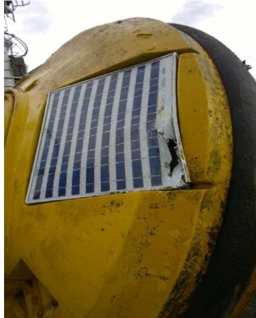
CALVAL – Solar panel damaged
