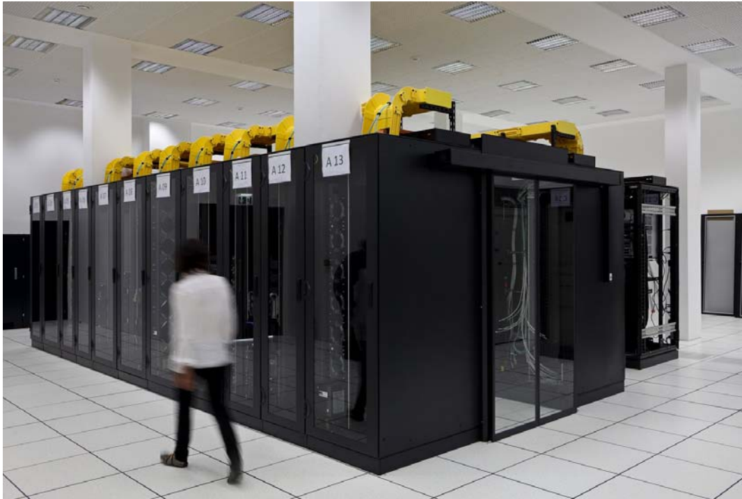
Figure 15 : CLS Global Processing Data Center
