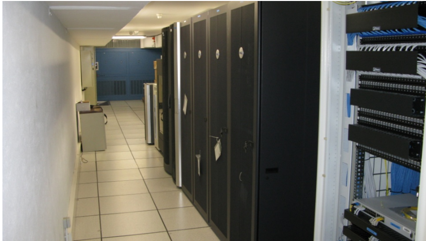
Figure 25 : Disaster Recovery Room located in CNES
