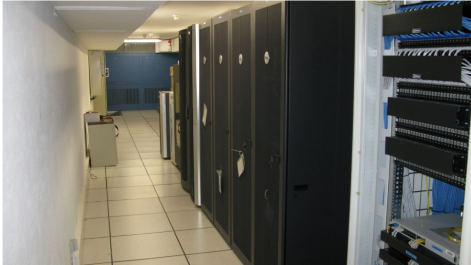
Figure 26 : Disaster Recovery Room located in CNES
