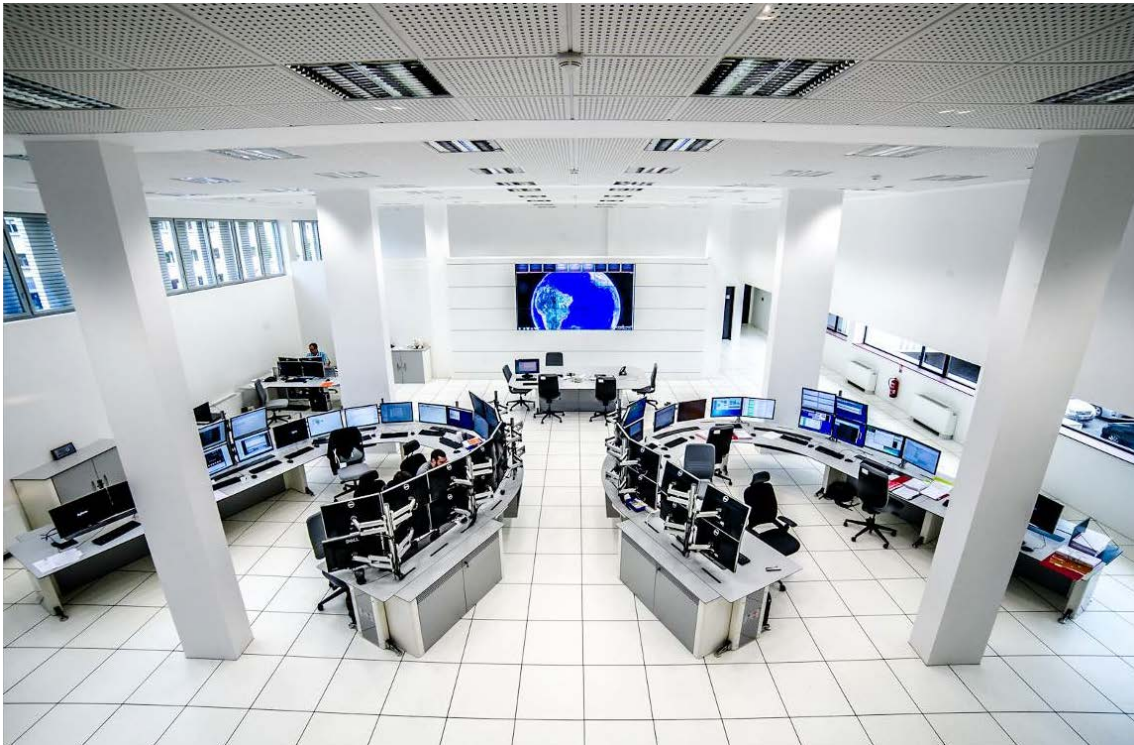
Figure 15 : CLS Toulouse Control Room
