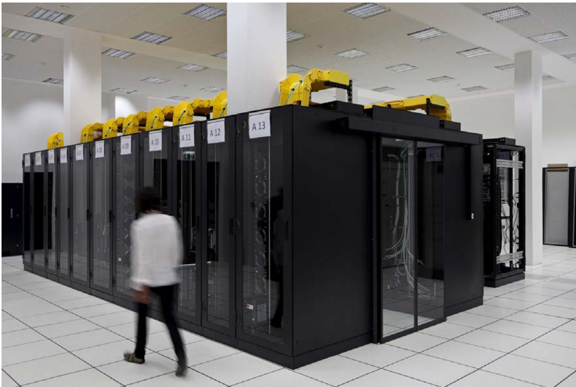
Figure 16 : CLS Global Processing Data Center
