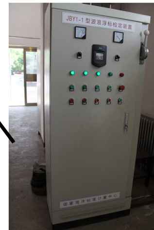
Frequency speed control and power supply system
