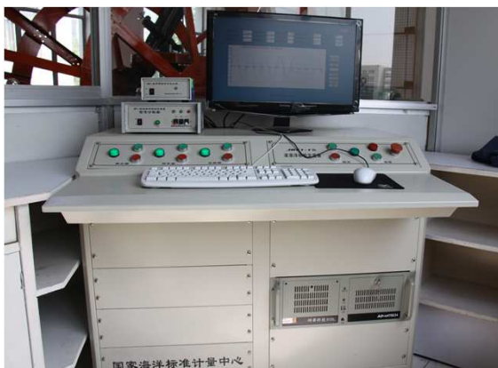
Control and data acquisition system
