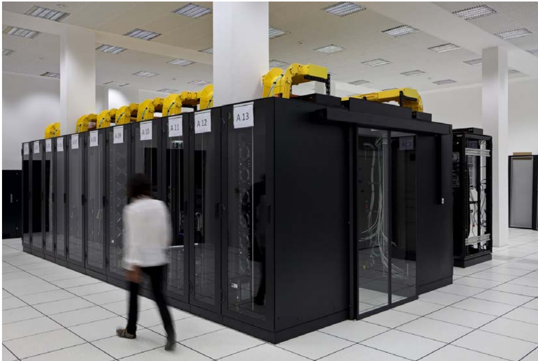
Figure 16 : CLS Global Processing Data Center
