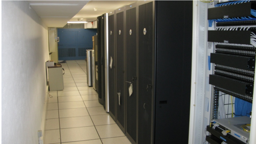
Figure 27 : Disaster Recovery Room located in CNES
