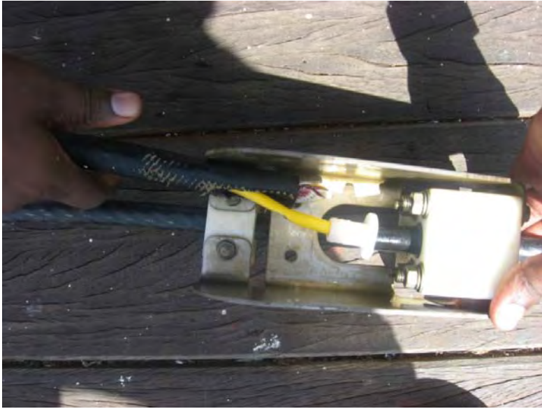
Damage in ICC Cable
