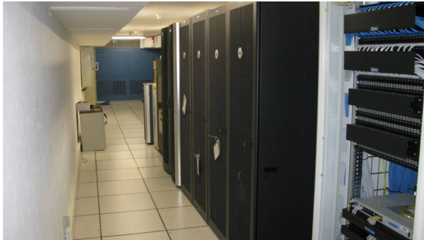
Figure 23 : Disaster Recovery Room located in CNES
