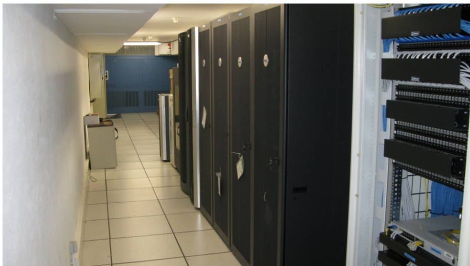
Figure 23 : Disaster Recovery Room located in CNES
