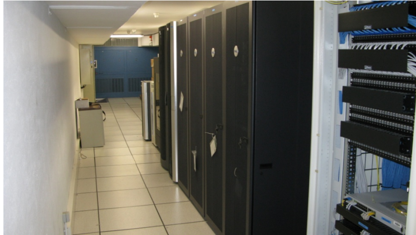
Figure 16: Disaster Recovery Room located in CNES (Toulouse, France)
