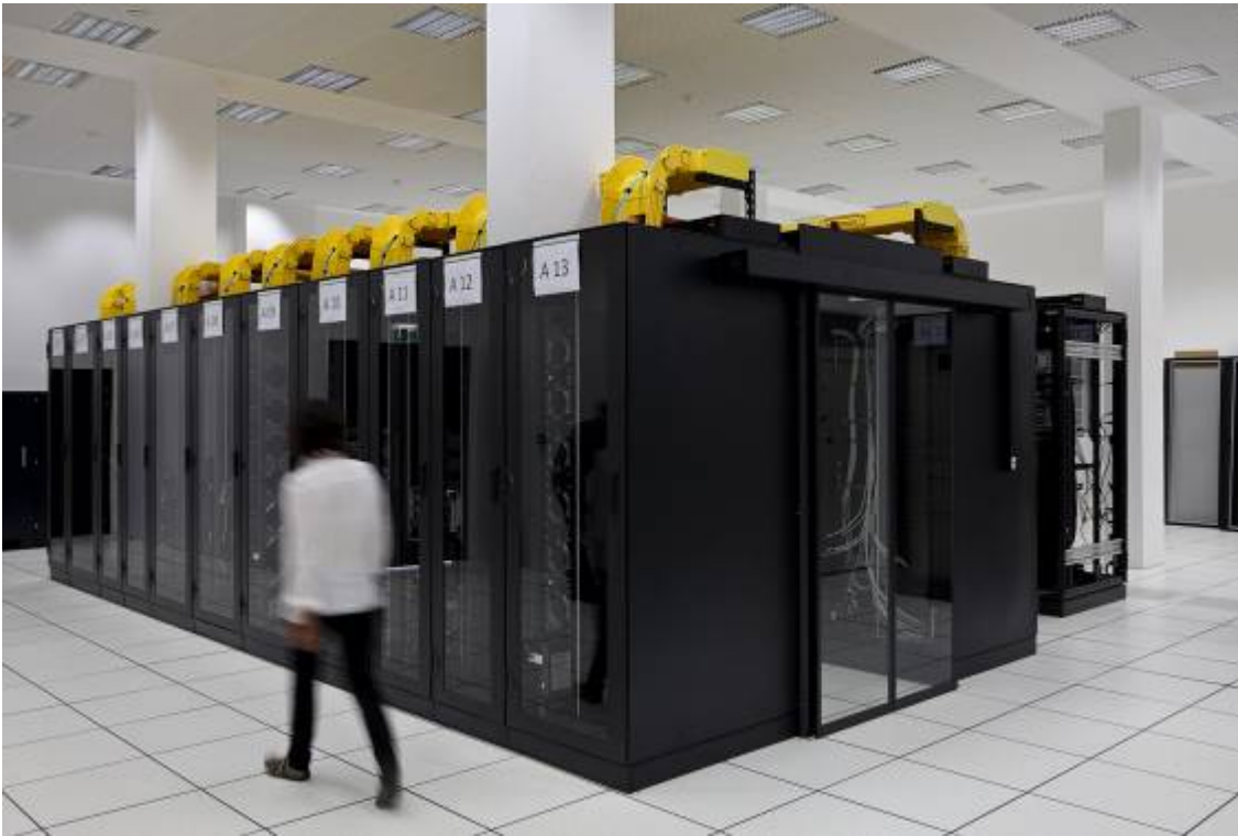
Figure 24 : CLS Global Processing Data Center
