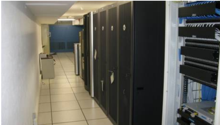
Figure 31 : Disaster Recovery Room located in CNES
