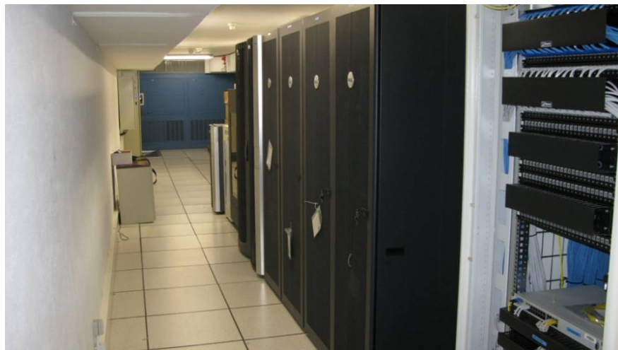
Figure 23 : Disaster Recovery Room located in CNES
