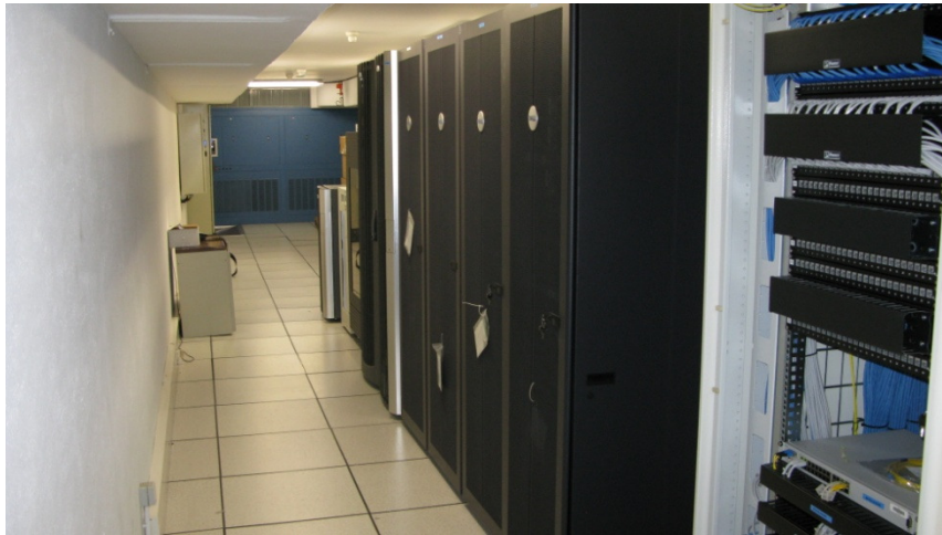
Figure 26: Disaster Recovery Room located in CNES (Toulouse, France)
