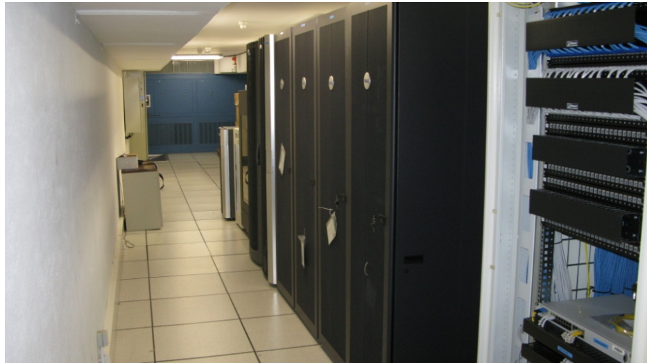
Figure 33 : Disaster Recovery Room located in CNES
