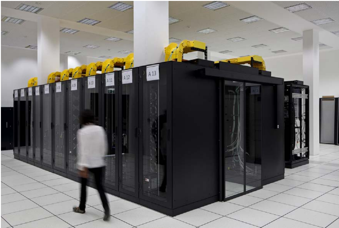
Figure 23 : CLS Global Processing Data Center
