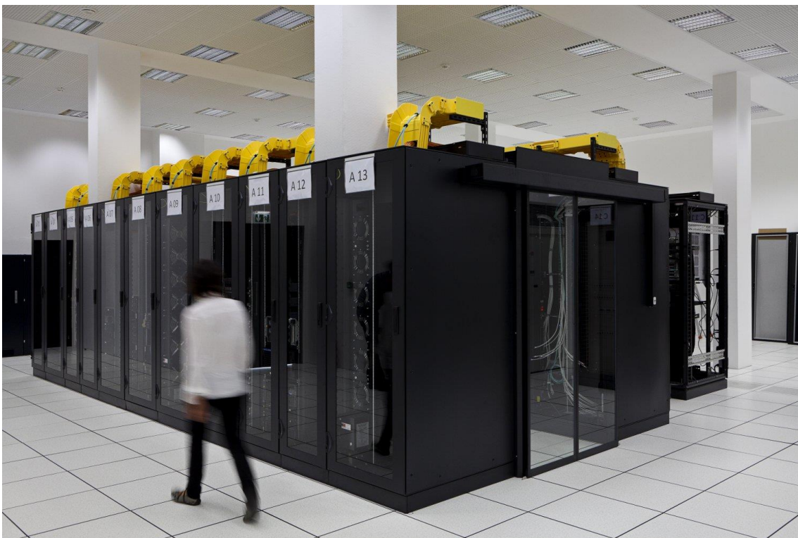
Figure 26 : CLS Global Processing Data Center
