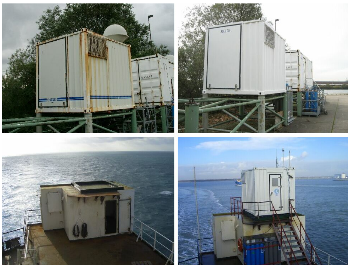
Figure 1: ASEU05 before and after refurbishment (upper left and upper right) and at installation on board the ATLANTIC COMPANION (lower left and lower right).
