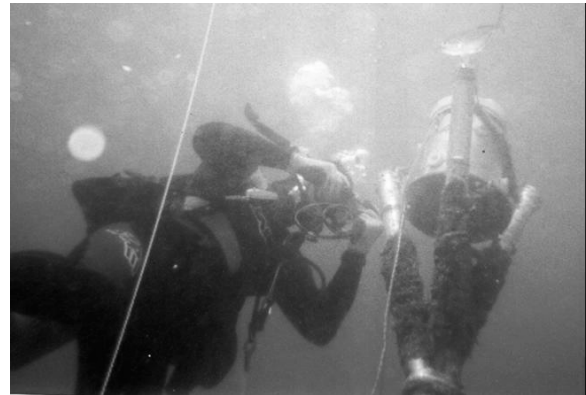
Figure 1 - Apex of tripod tower, showing ADCP wave instrument.
